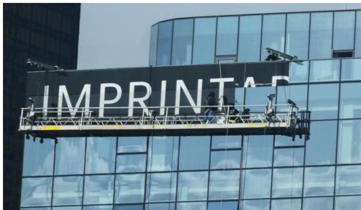
Trying to make a good first impression. Imprint Apartment building at 717 S Clark. Photo Oct 20, 2020.
