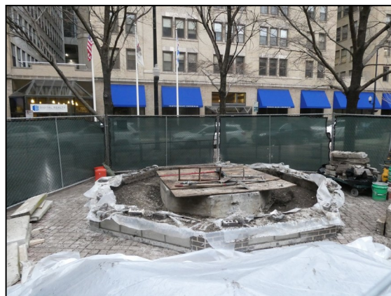
The New rehabbed fountain in Printers Row Park is being installed as we speak.
